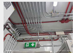
➢ Secondary Wiring on Indoor Top
