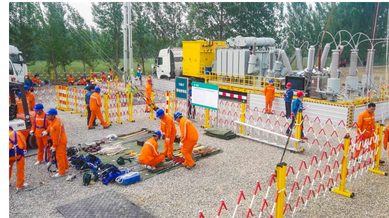
> State Grid Shandong 110 kV Mobile Trailer Substation
