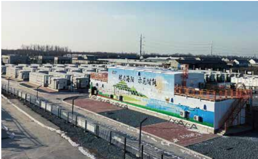
✔ Energy storage industry
