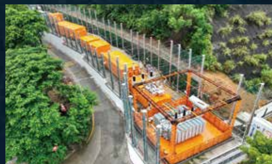
Substation load transition
