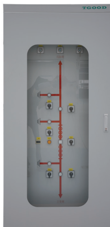
Local control cubicle
