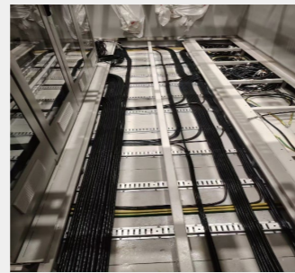
> Secondary Wiring on Indoor Floor
