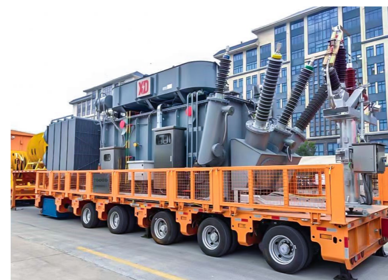
> Guangxi Hezhou 110 kV Mobile Trailer Substation
