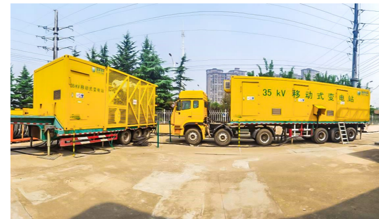
> Shandong Qingdao 35 kV Mobile Trailer Substation
