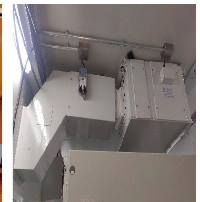
Wall-mounted Integrated Fan
