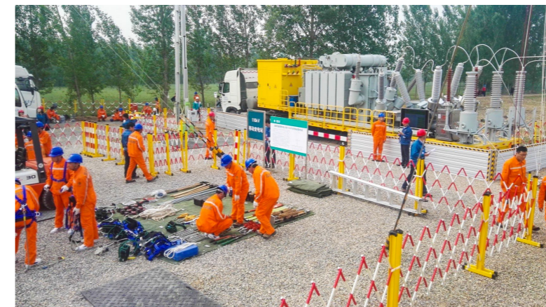
> State Grid Shandong 110 kV Mobile Trailer Substation
