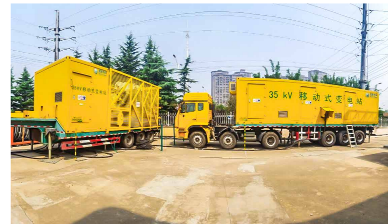
> Shandong Qingdao 35 kV Mobile Trailer Substation
