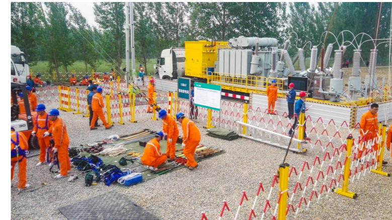
> State Grid Shandong 110 kV Mobile Trailer Substation
