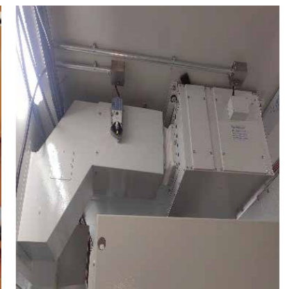
Wall-mounted Integrated Fan
