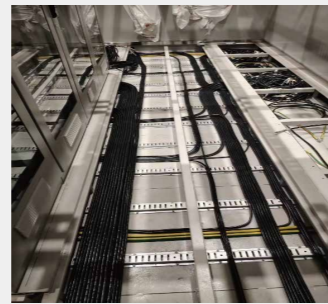
> Secondary Wiring on Indoor Floor
