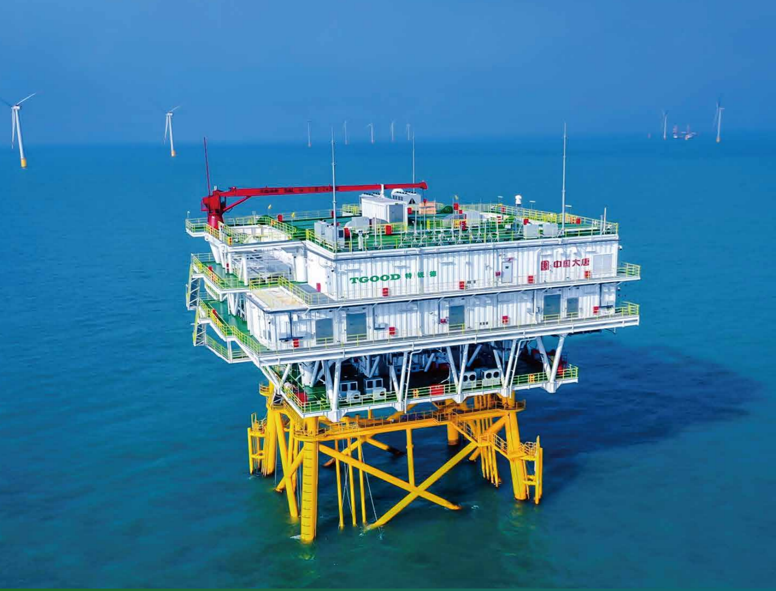
CHINA 220/35KV OFF-SHORE PREFABRICATED SUBSTATION
