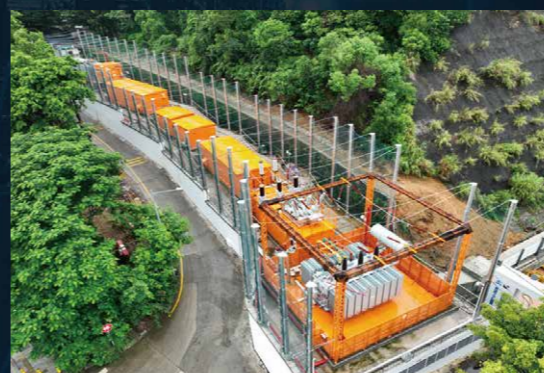
Substation load transition
