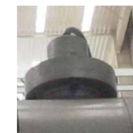
Electronic current transformer
