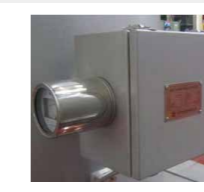
Surge arrester online monitoring sensor
